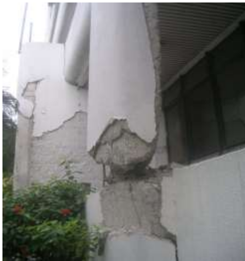
Fig. 4b: Damage of the column base ( http://db.concretcoalition.org/building/144 )
