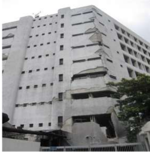
Fig. 4a: Exterior damage to the teleco building, Haiti
