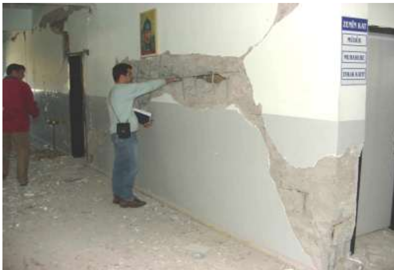
Fig. 3b: Concrete crushing in shear wall due to Bingol 2003 Earthquake ( http://db.concretecoalition.org/building/133 )
