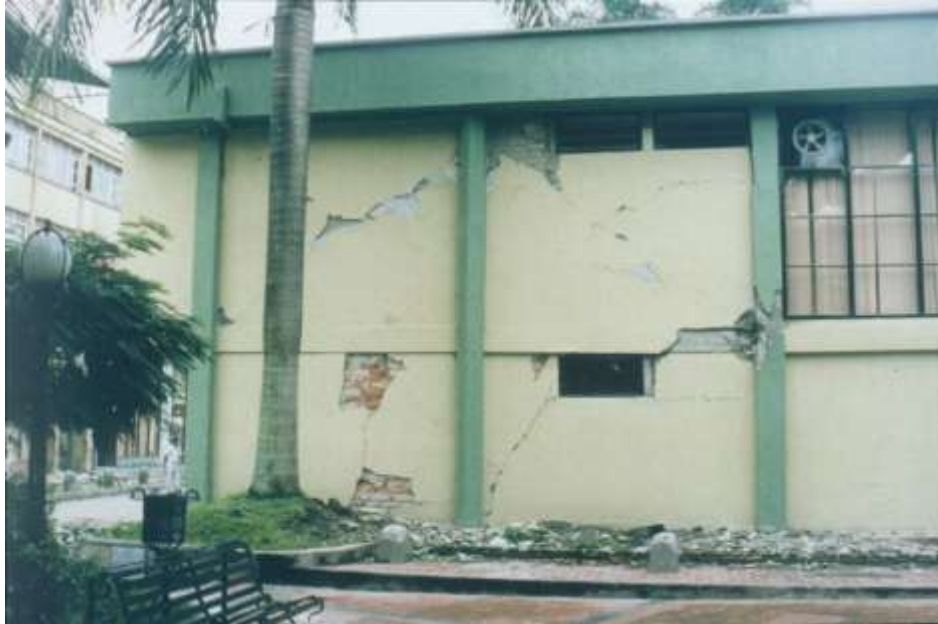
Fig. 2: Municipal building in Armenia, Colombia ( http://www.ngdc.noaa.gov/hazardimages/picture/show/824 )
